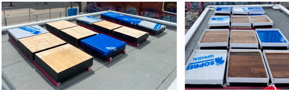
Fig. 3. 4-month exposure period (left), and 2-month bulk water inundation period (right).
